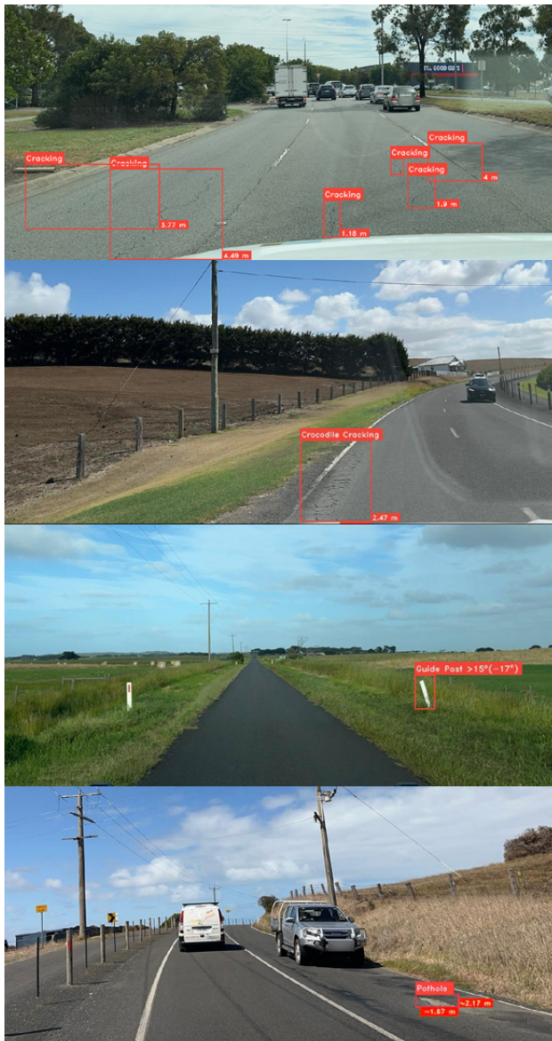
Example AI detected defects
